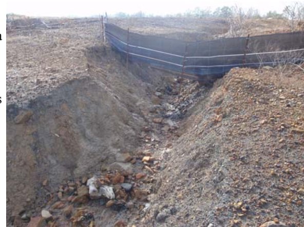
This Gardendale construction site has erosion gullies so deep that you can almost walk under the silt fence. Photo by Nelson Brooke.
