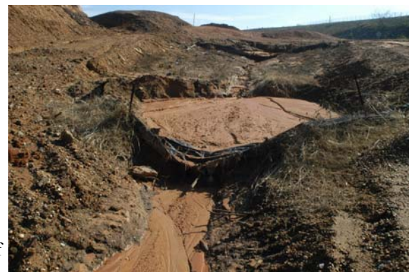
Poor erosion controls at this Tuscaloosa site render silt fences useless and allow incredible amounts of sediment to flow into nearby streams. Photo by Nelson Brooke.
