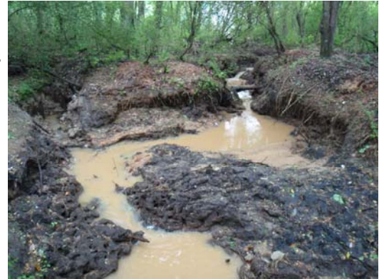
A Northport construction site's pollution. Photo by Nelson Brooke.
