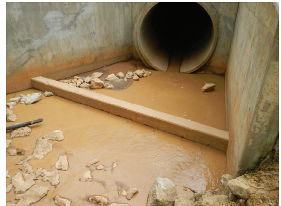
Even on this non-rain day, muddy water flows from UA's new stormwater pipe which drains the new part of campus uphill of Manderson Landing at River Road Park.
