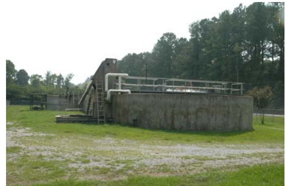
4,473 Clean Water Act Violations East Walker Co. Wastewater Treatment Plant © Nelson Brooke 2005
