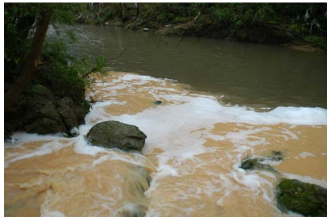
Turbid water and foam from the Airport expansion pollutes Village Creek after a rain. © Nelson Brooke
