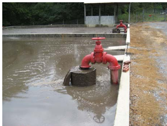
Riley Maze Wastewater Treatment Plant in Arab, AL discharges improperly treated wastewater to Riley Maze Creek, prompting legal action. © John Kinney
