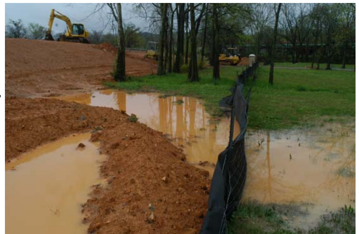
This project lacks adequate erosion control measures, and its silt fences have failed to stop sediment from running off site.
