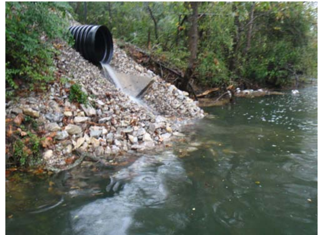
Birmingham Hide & Tallow's new pipe discharging into Valley Creek in Bessemer. Photo by Nelson Brooke.
