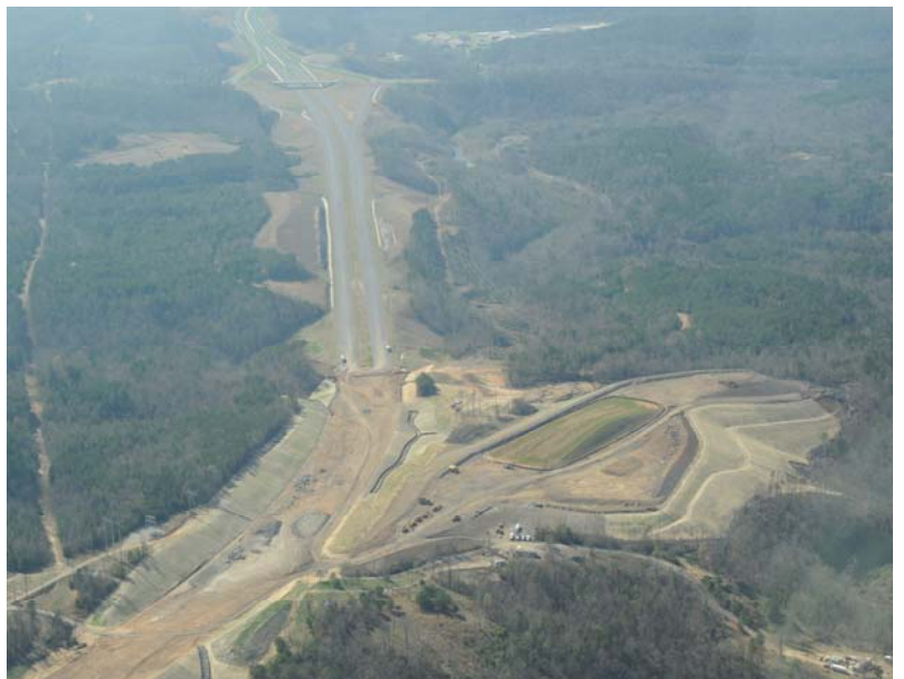
Aerial view of ALDOT's Corridor X (I-22) construction nearing its final junction at I-65 in Birmingham.
