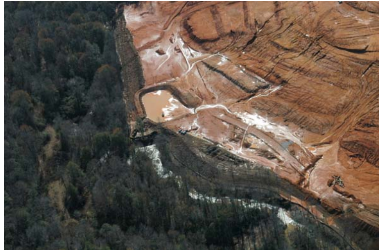
Badly eroding construction site polluting a creek in the Mill Creek watershed, West of Northport.
