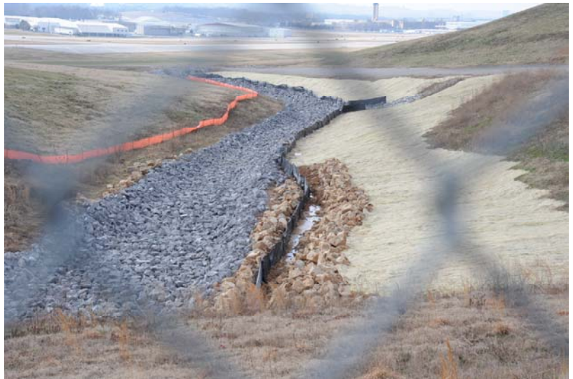
Additional erosion control measures were added to this drainage at the Birmingham Airport in response to our case settlement. Photo by Nelson Brooke.
