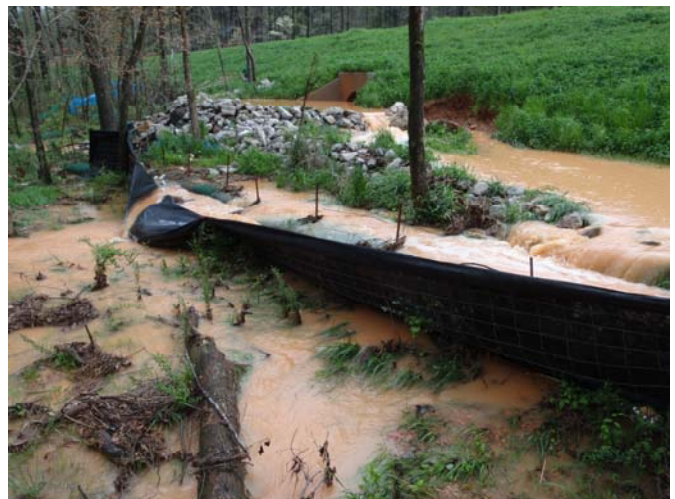
Muddy water spills out of Bessemer High School's construction site. Photo by Nelson Brooke.
