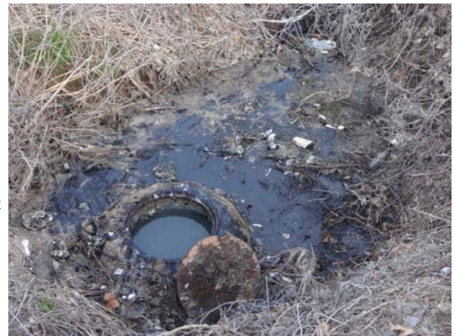
Sewage overflow at a manhole in Hueytown. This sewage flowed into Opossum Creek, a tributary of Valley Creek — a major recreation spot in Jefferson County.
