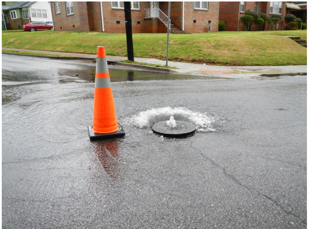
Sewage flows from a Birmingham manhole, enters a nearby storm drain, and eventually flows to Village Creek, a major tributary of the Black Warrior River's Locust Fork in Jefferson County. Photo by Nelson Brooke.
